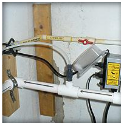
Solution injector and flow switch for chlorine feed pump system.
