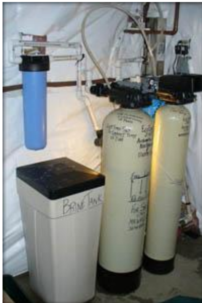
Well Water System
