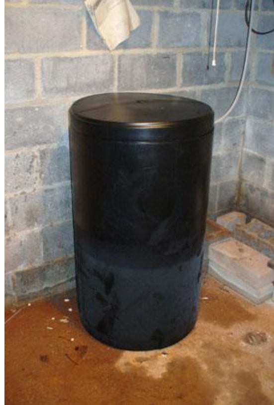
Salt Tank for 120,000 grain Water Softener
