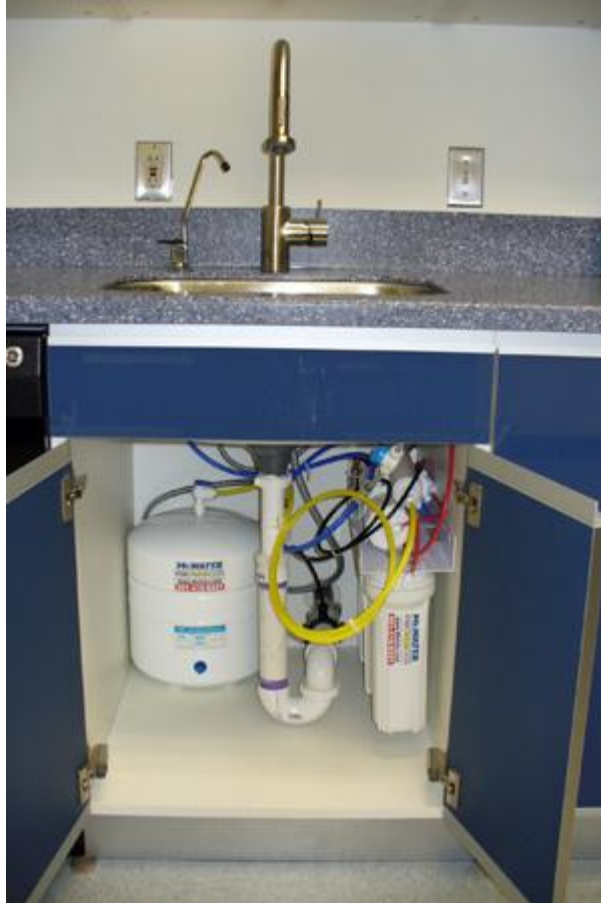
Standard 5 Stage Reverse Osmosis System - commercial under sink installation
