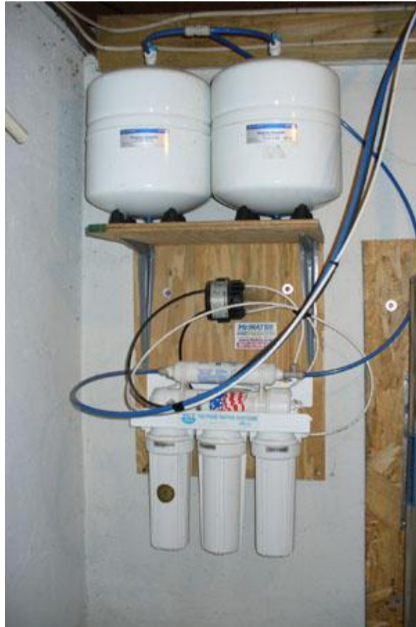
5 Stage Reverse Osmosis System with Permeate Pump and Dual Storage Tanks - basement installation
