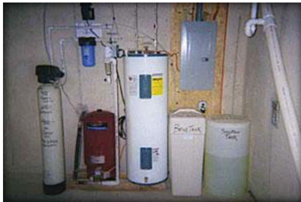
EcoSoft Water Treatment Systems™ Water Softener and Stenner® peristaltic chemical feed pump system treating hard water conditions and sulfur (rotten egg) smell in Berkeley Springs, WV 25411.
