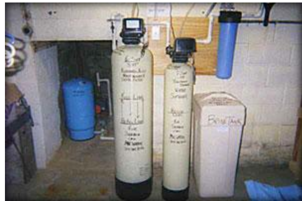
Heavy Duty Acid Neutralizer and Depth Filter with Water Softener and Carbon Filtration for petroleum byproducts. Installed in Mt. Airy, MD 21771.
