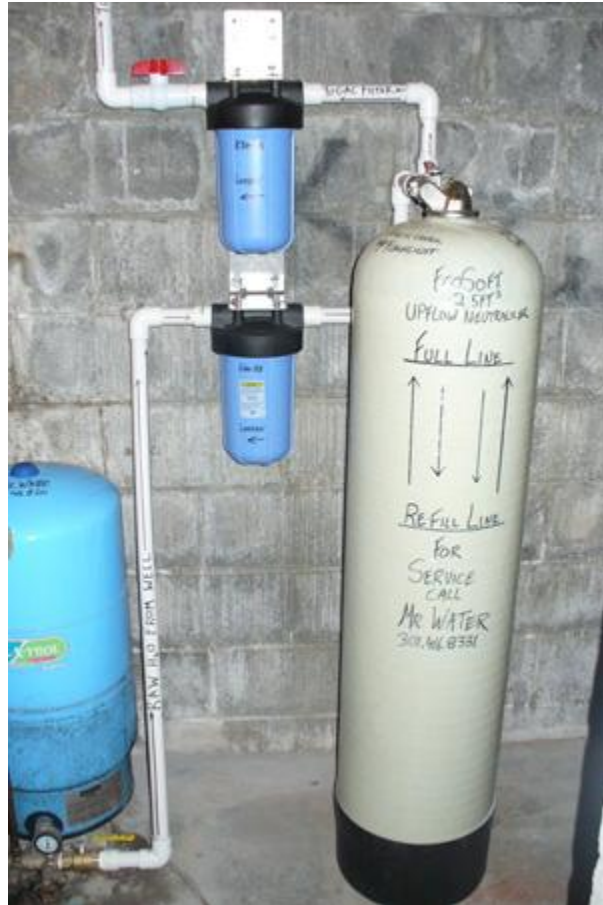
2.5 cubic foot Up Flow Acid Neutralizer
